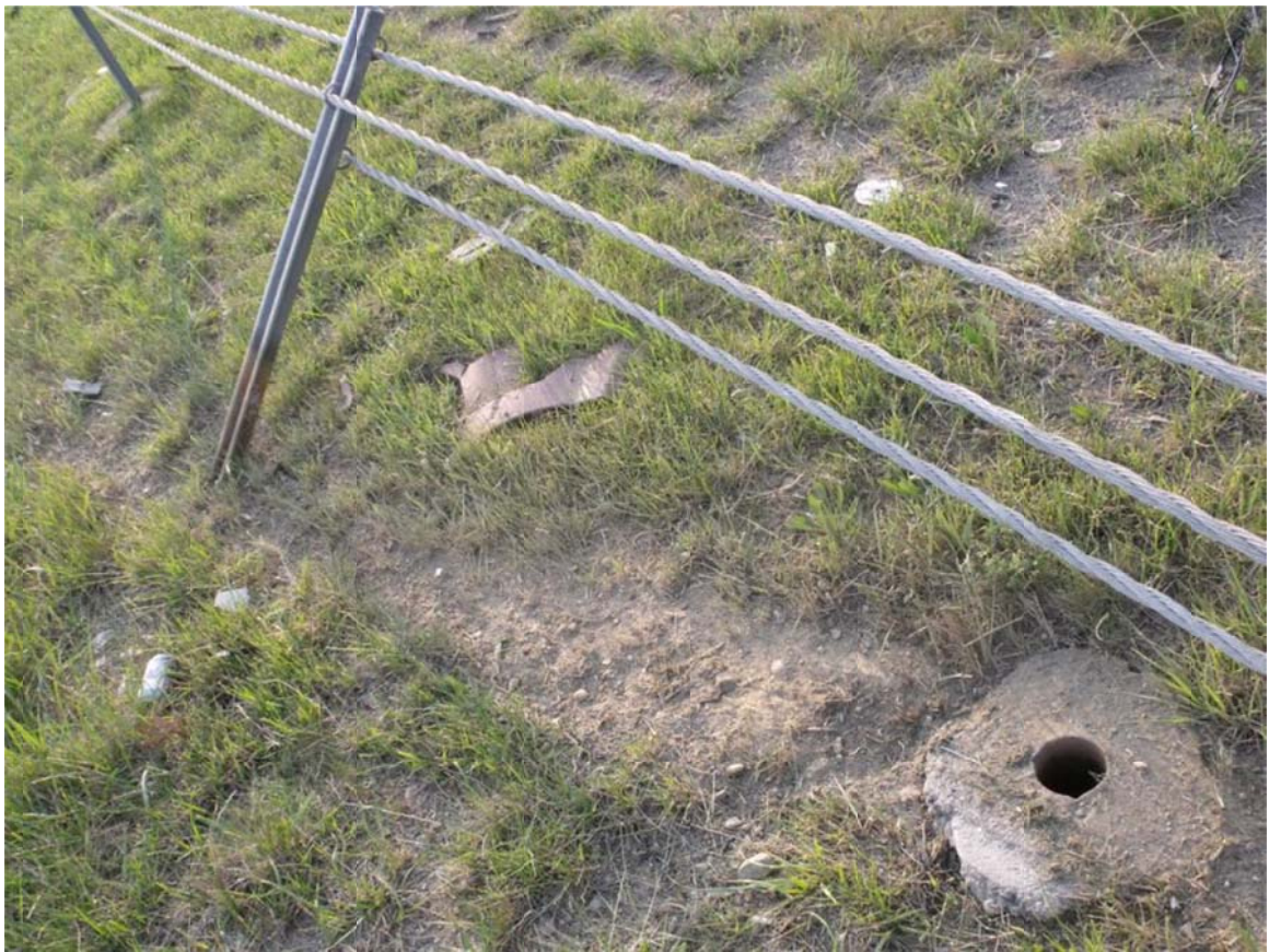
Figure 85. Prying Penetration Crash on Nucor NU-CABLE Barrier
