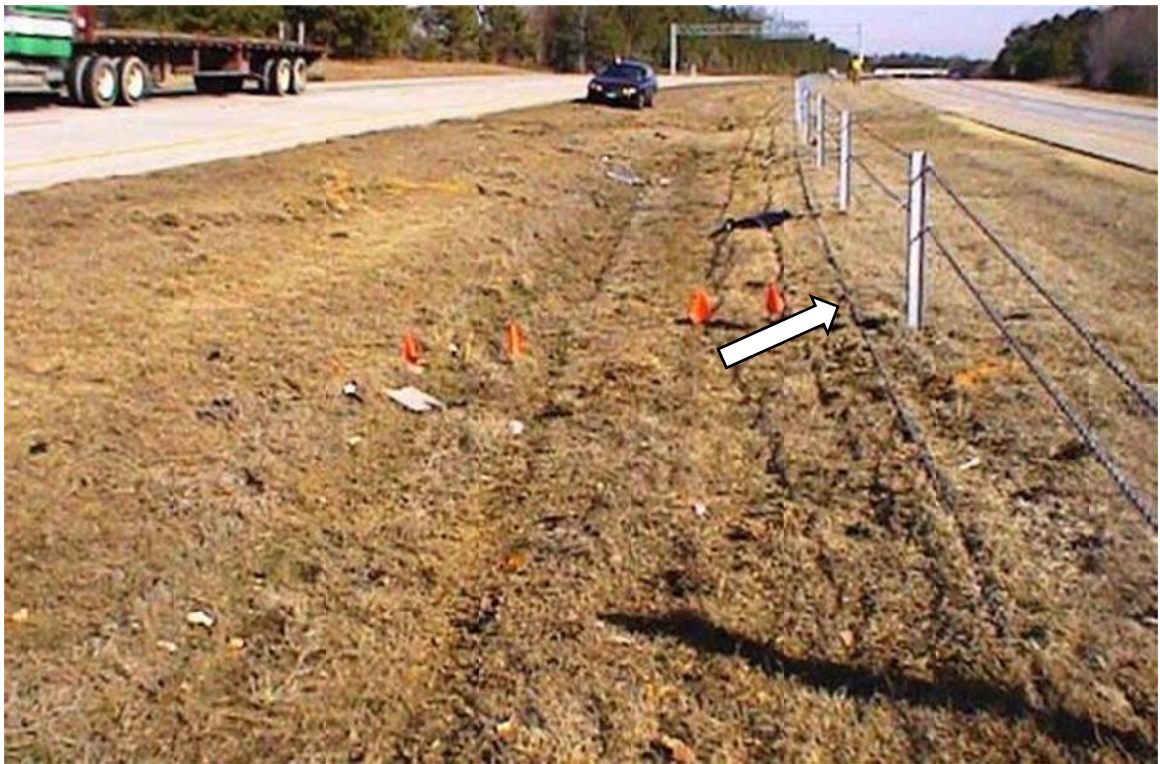
Figure 99. Back Side (Middle) Cable Release from 11 Downstream Posts Resulting in Penetration
